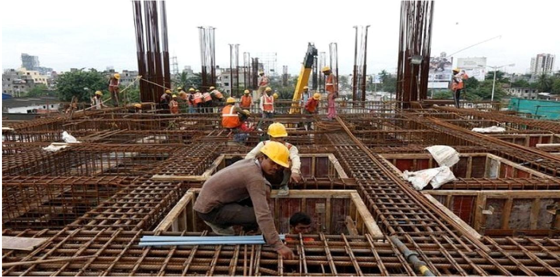
Figure 1. Typical ergonomic and occupational hazards observed at a construction site, including awkward postures, manual material handling, and repetitive tasks [9]
